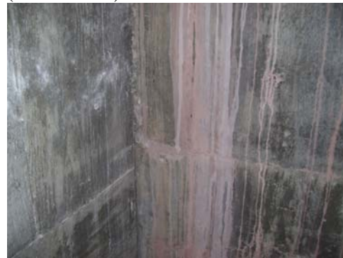
Office Area, COTC Side (Adult Ed) – mold growth not observed on concrete wall; whitish areas are due to moisture infiltration (efflorescence)
