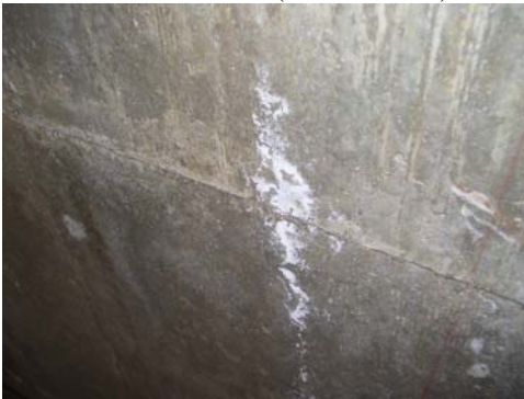
Laboratory Area (Adult Ed) – mold growth not observed on concrete wall; whitish areas are due to moisture infiltration (efflorescence)
