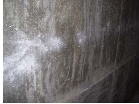
Office Area, COTC Side (Adult Ed) – mold growth not observed on concrete wall; whitish areas are due to moisture infiltration (efflorescence)
