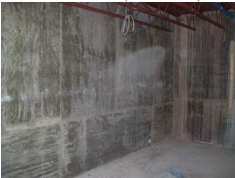
View of exposed concrete wall systems in Office Area, COTC Side (Adult Ed)
