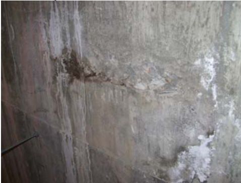
Laboratory Area (Adult Ed) – mold growth not observed on concrete wall; whitish areas are due to moisture infiltration (efflorescence)
