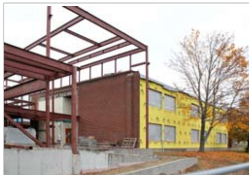
Steel goes up for the new library and administrative wing, as the exterior of the first classroom wing awaits masonry.
