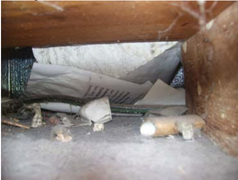
Room 105 – accumulated dust and debris under heating unit
