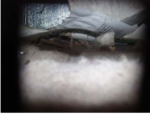
Room 105 – accumulated dust and debris under heating unit
