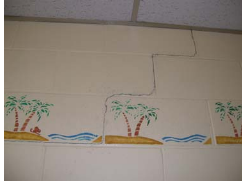
Room 208 – crack in wall (example of pathways that may allow airflow and particulates to enter a classroom)
