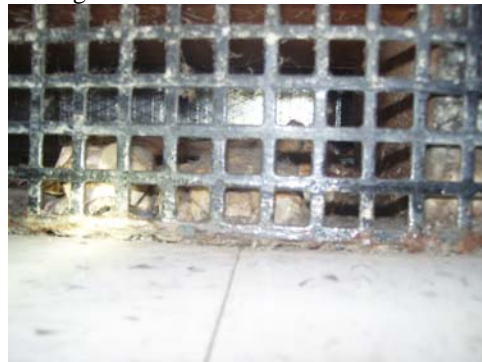
Room 223 – accumulated dust and debris under heating unit
