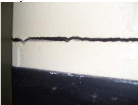
Room 208 – large crack in wall (example of pathways that may allow airflow and particulates to enter a classroom)
