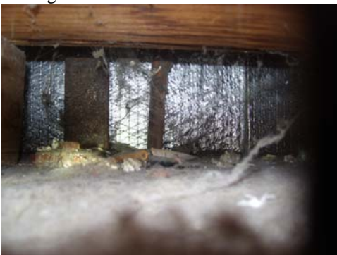
Room 115 – accumulated dust and debris under heating unit
