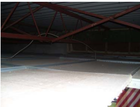
Room 215 / 216 area above ceiling tiles – no mold / moisture issues noted, residual dust typical for type of space
