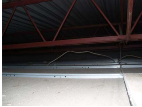
Room 215 / 216 area above ceiling tiles – no mold / moisture issues noted, residual dust typical for type of space
