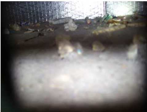
Dust and debris accumulated under the heating unit in Room 203
